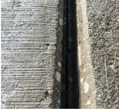
Figure 3 Photo of Wet Saw Joint Condition After Power Washing and Vacuuming
