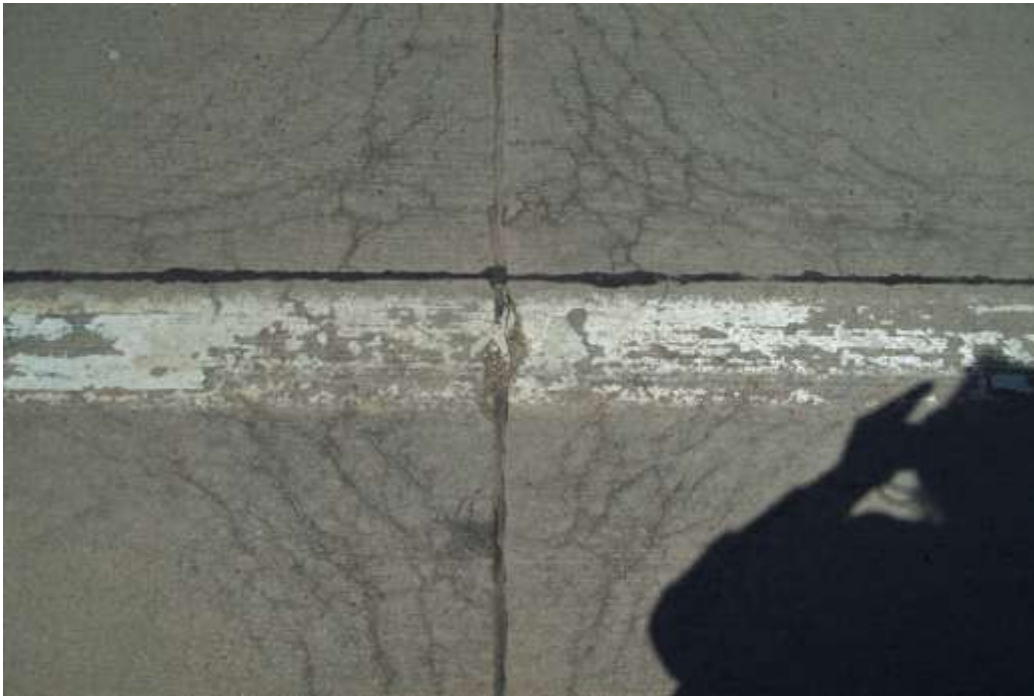
Photo 2: ASR cracking in a Mid-west pavement containing reactive quartzite coarse aggregate.
