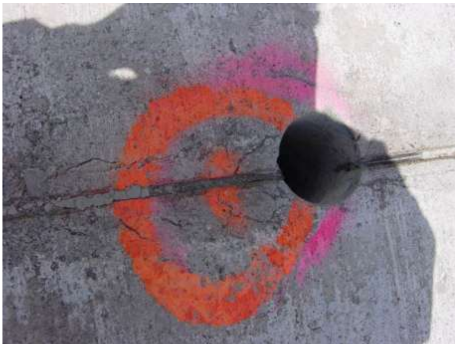
Photo 7: Pavement joint compromised by premature saw-cutting. Note tears/deformation in the surface paste.
