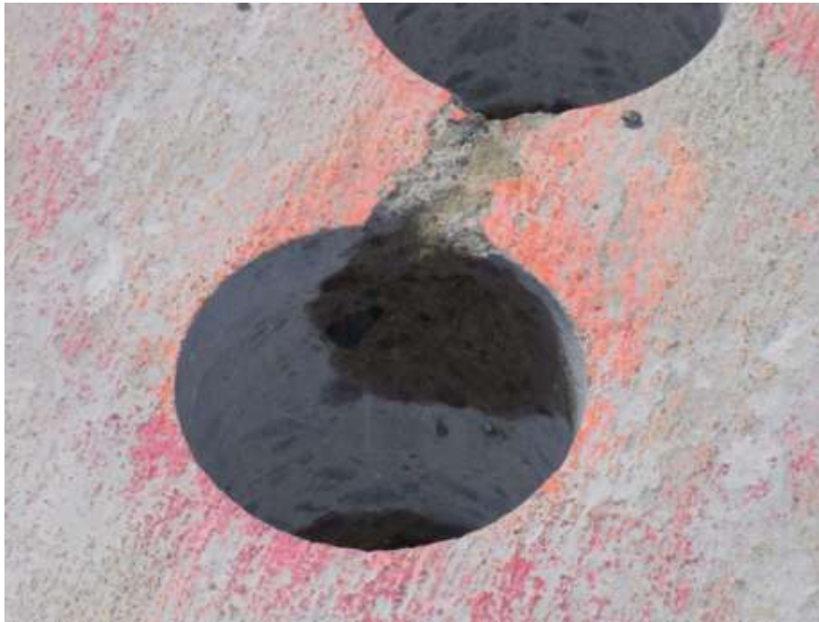
Photo 8: Incomplete mixing in concrete pavement. Note raveled and saturated mass of concentrated flyash; core-sampled for analysis.
