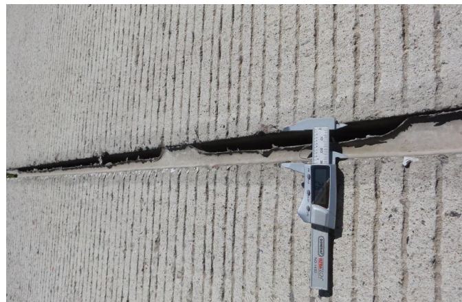
Figure 7. Adhesive failure on longitudinal joints.
