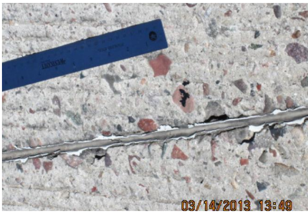
Figure 2. Spall failure – transverse joint (section 264).
