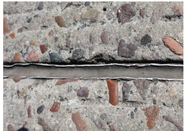
Figure 5. Adhesive failure – transverse joint (sect. 215)
