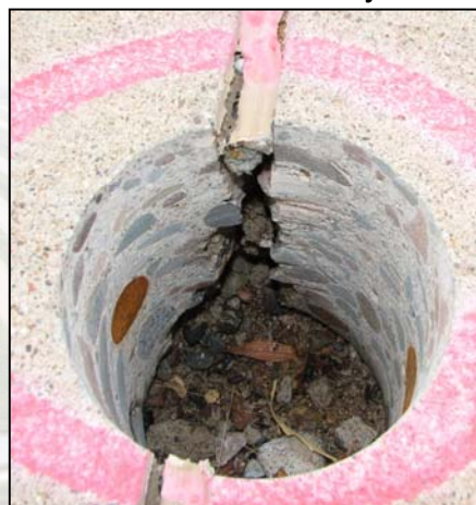
Photo 2. Effect of breached joint seal.
